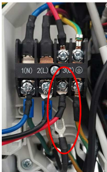
IDU terminal block wiring
